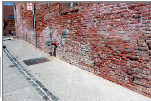
A doorway that was bricked-in, showing that the street had been filled in and the original floor level was much lower.
